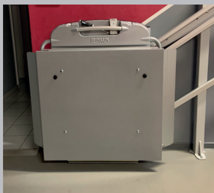
Platformslift lige trappe
